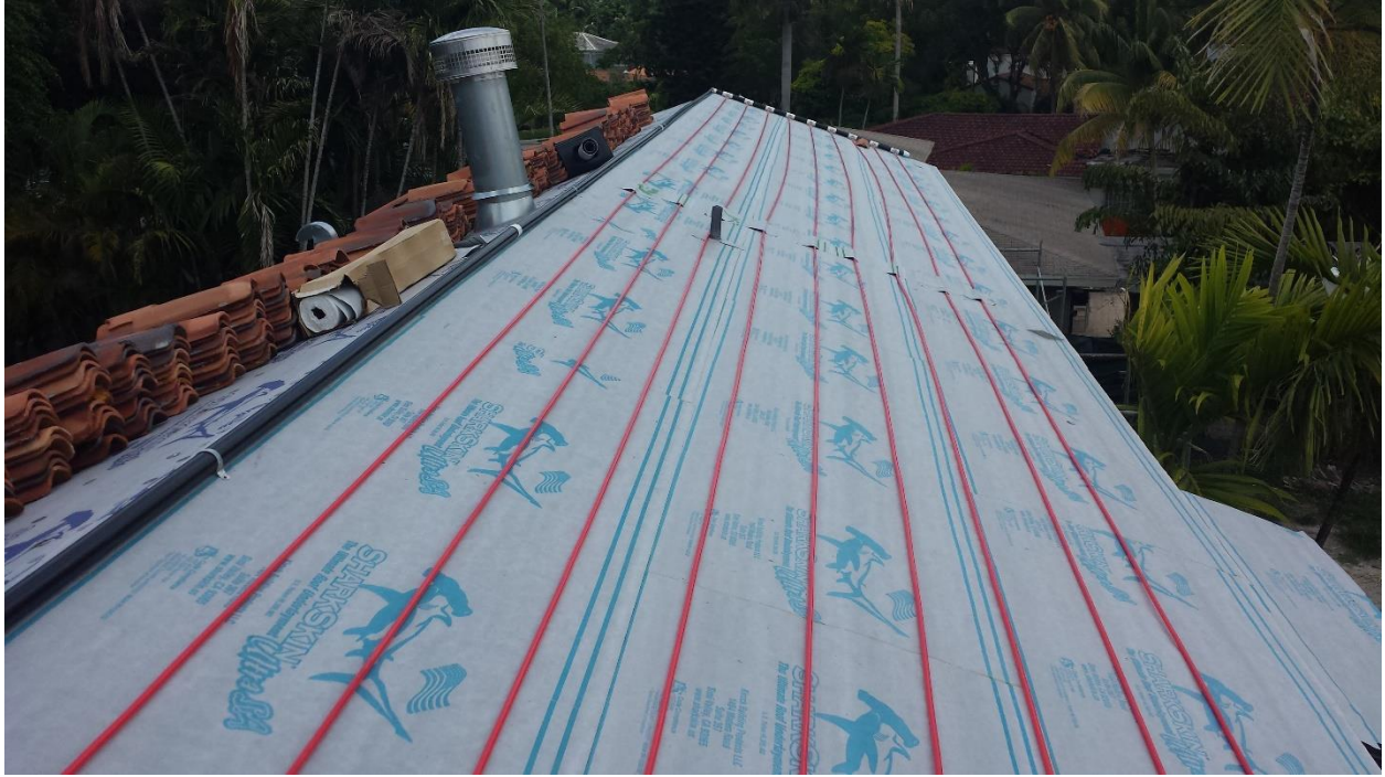
Second story view “Invisible Solar Thermal” ArteZanos® Roof Integrated Solar Absorber (R.I.S.A.) tubing in City of Miami Historic District Courtesy of ArteZanos® 2014
